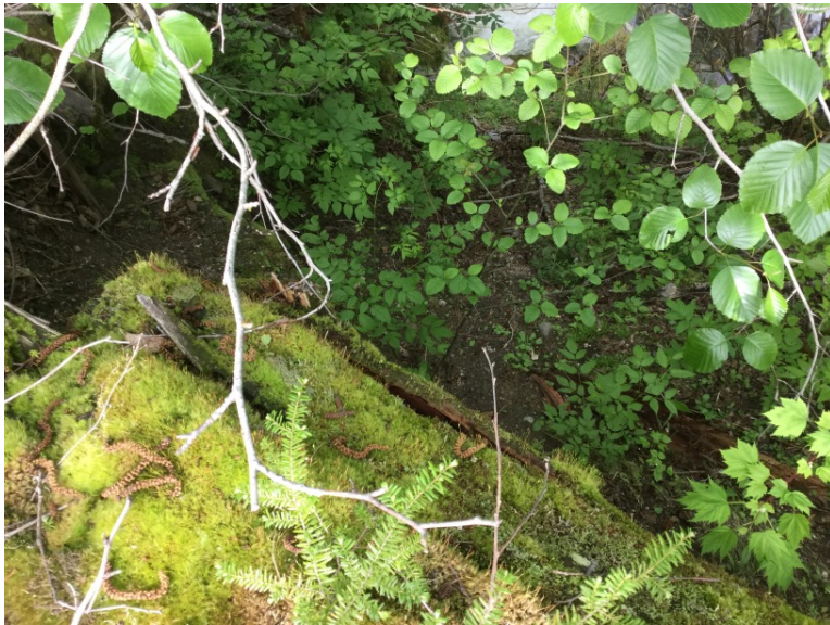
Eroding fill slope at downstream right bank
