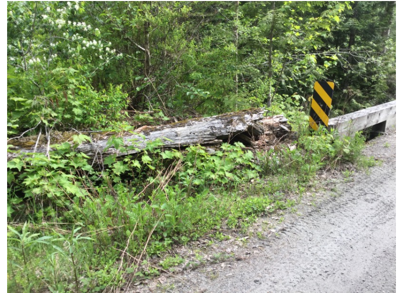
Log fender condition
